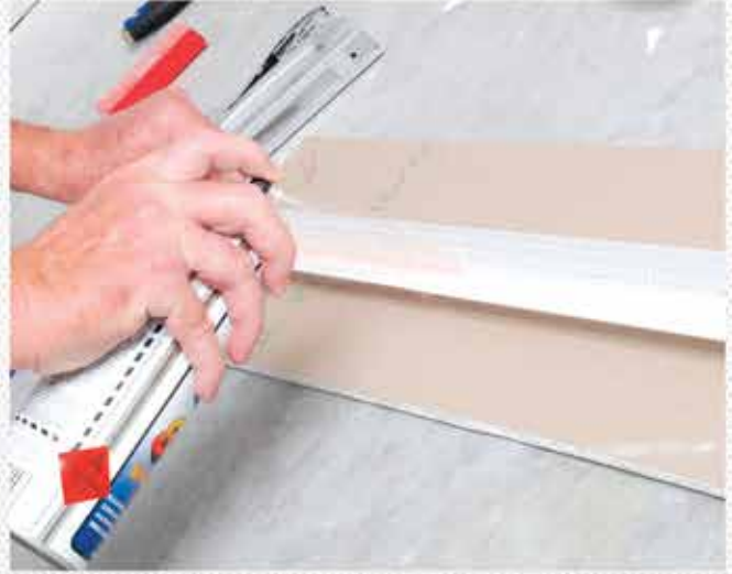
2. Spray a liberal coat of Trim-Tex 847 Spray Adhesive to the inside of the bead and the surface of the plasterboard
